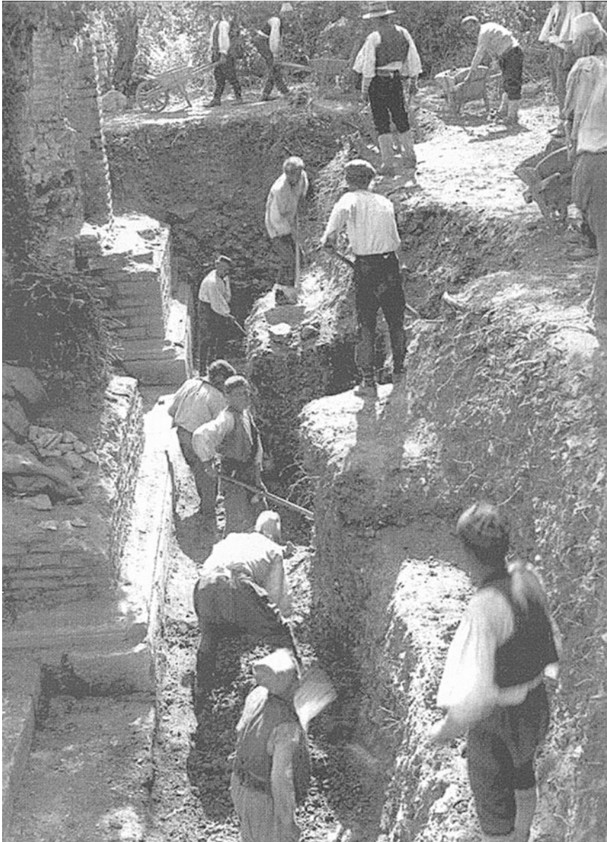
Fig. 12. Ugolini's excavation trench adjacent to the scaenae frons , 1928 (courtesy of the Butrint Foundation).
